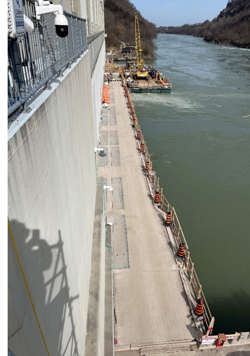
A look at the new tailrace deck at the Sir Adam Beck I hydro station in Niagara Falls.
