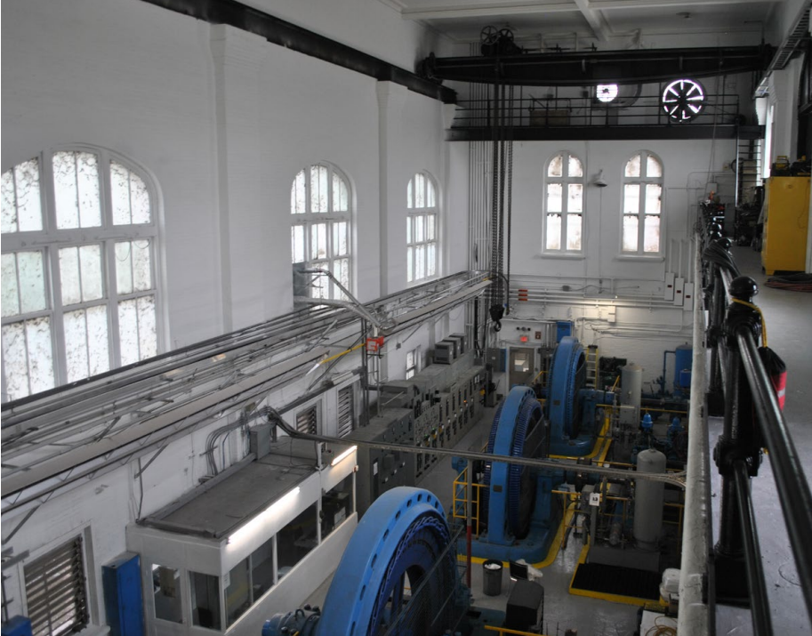
Figure 25: London Street Generating Station Plant #1 (4 MW) and new Plant #2 (6 MW)
