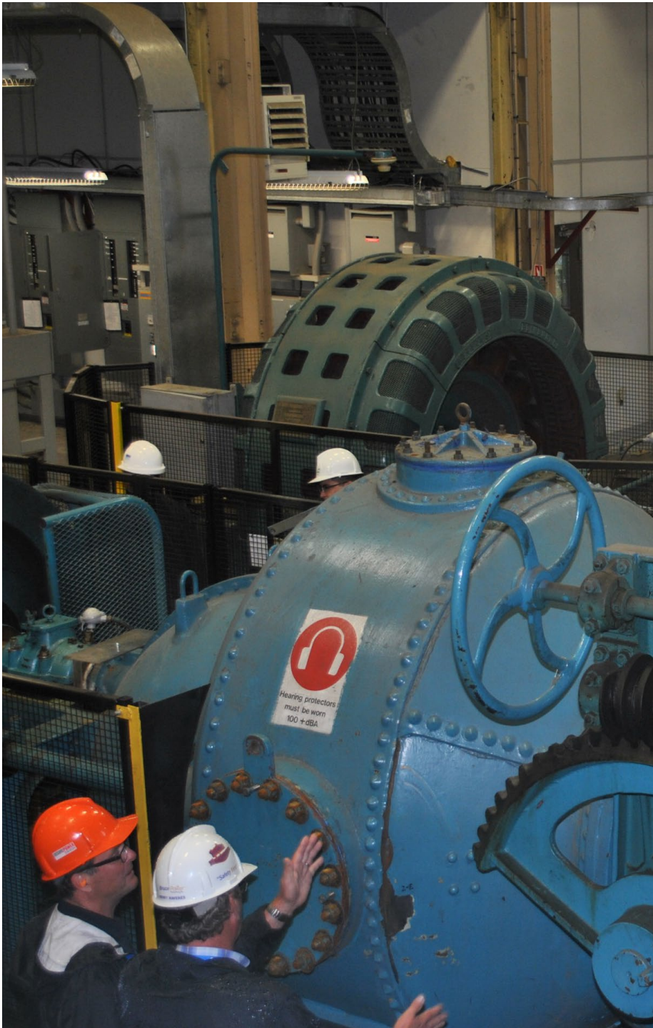
Figure 18: South Falls Generating Station, located in Muskoka, Ontario - Ontario Power Generation (5 MW)
