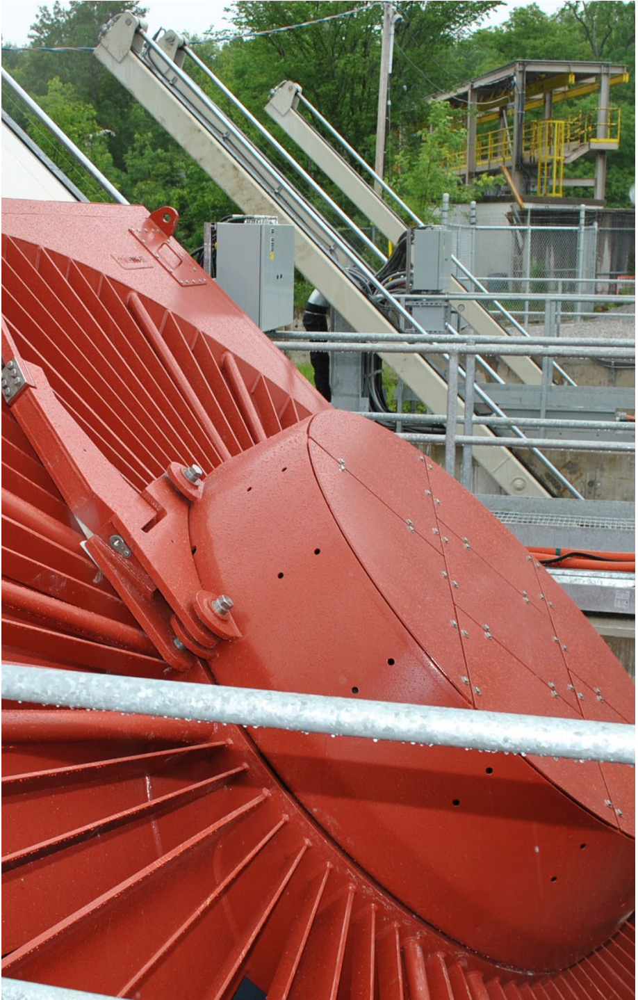
Figure 24: Wasdell Falls Generating Station (1.65 MW) - Wasdell Falls Limited Partnership (WFLP) - Very Low Head (VLH) Turbine
