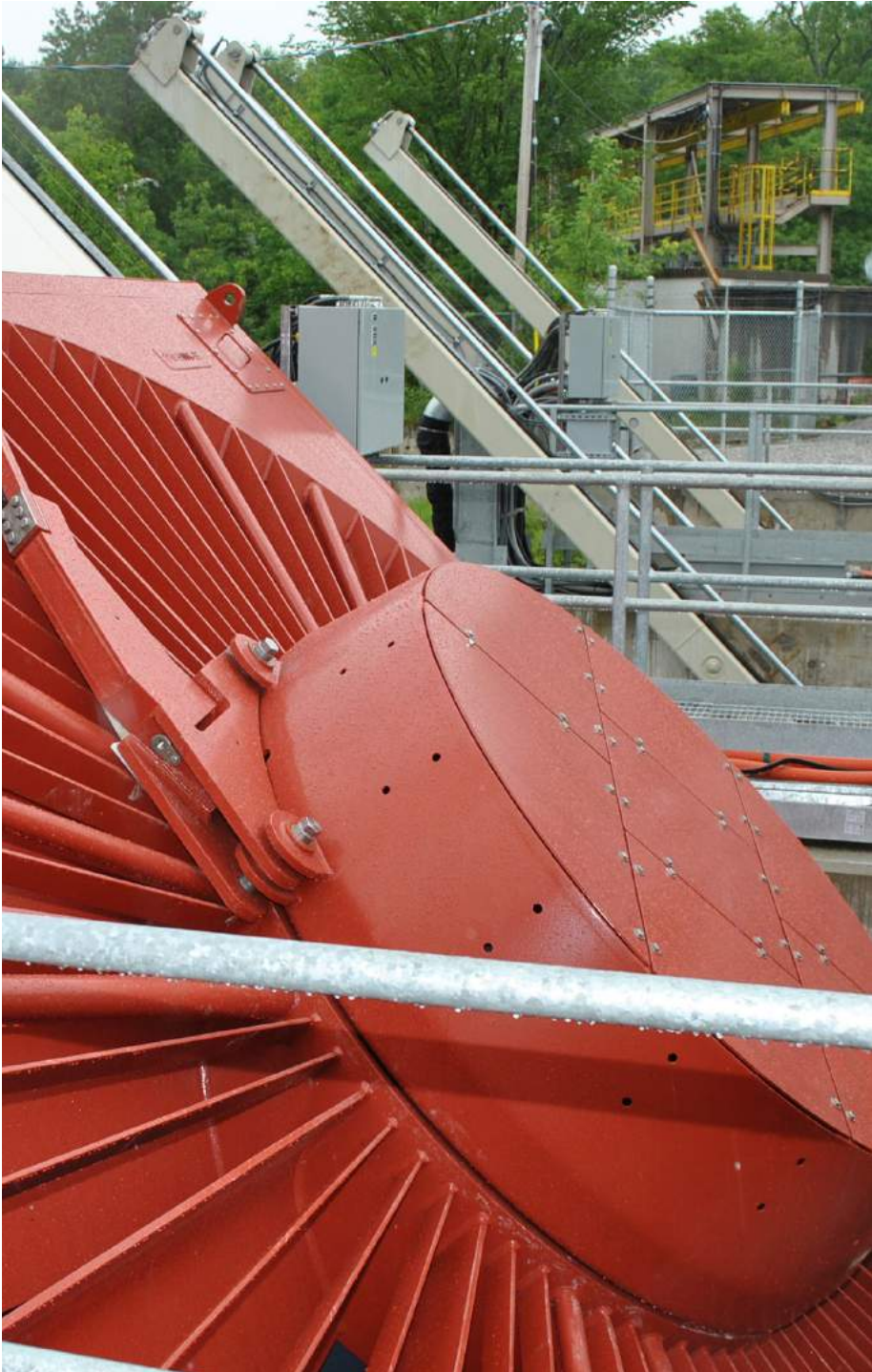
Figure 27: Wasdell Falls Generating Station (1.65 MW) - Wasdell Falls Limited Partnership (WFLP) - Very Low Head (VLH) Turbine
