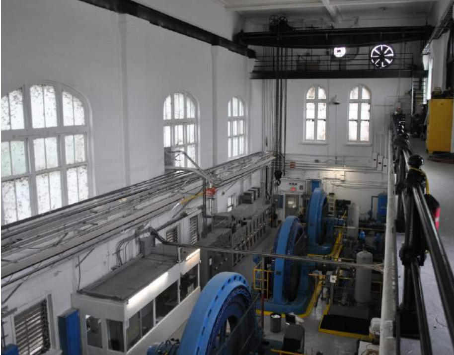
Figure 28: London Street Generating Station Plant #1 (4 MW) and new Plant #2 (6 MW)
