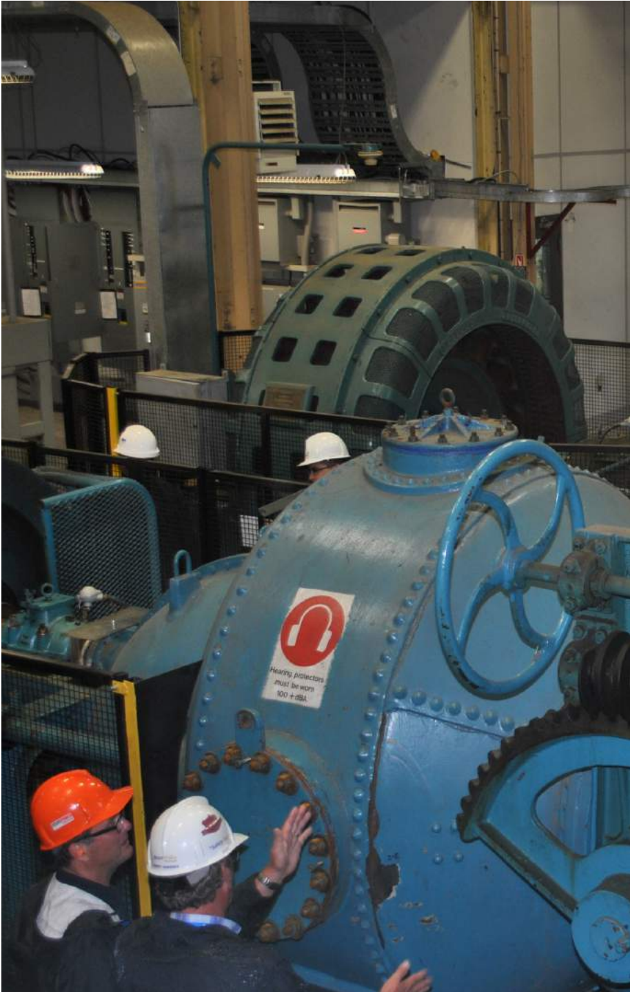
Figure 21: South Falls Generating Station, located in Muskoka, Ontario - Ontario Power Generation (5 MW)
